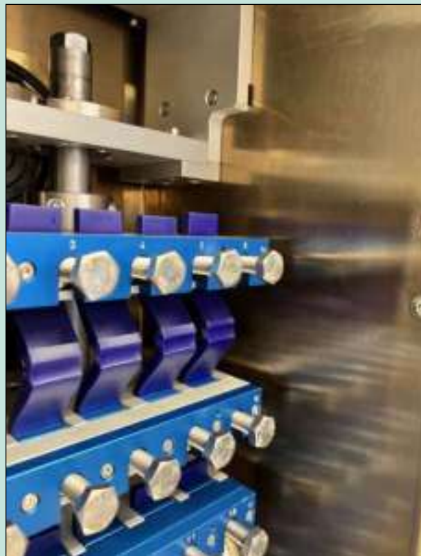
Figure 2 - temperature control via an integrated refrigeration unit
