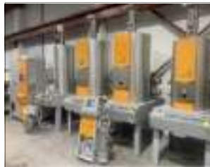
4 Hopper Motan dehumidifying system
