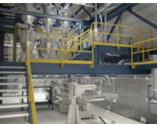
Greenfield & New Equipment
